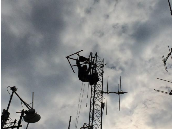
Tower worker and engineer Derek Jackson puts the finishing touches on the new KLZ-FM antenna installation.
