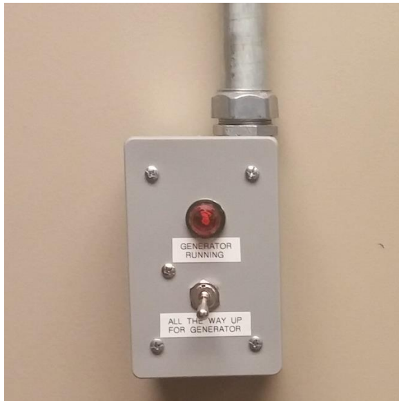
Figure 1 - Manual switch to force generator operation.
