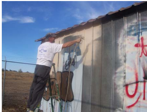
It's bye-bye graffiti at the KLZ barn. Note the new fence in the background.
