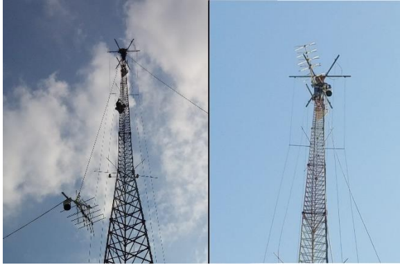
Figure 2 - Left: the antenna and mount headed up; right: the antenna in place.
