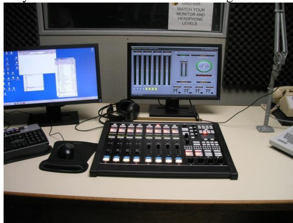
New Wheatstone E6 control surface in KBRT Prod E. One other production room at KBRT will get an E6 as part of the WNIP project there.
