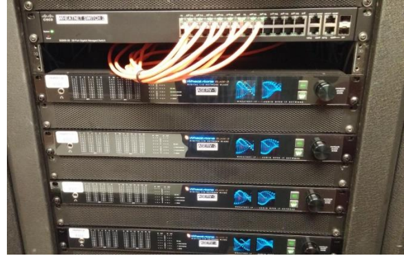
Figure 2 - The blades for the Audio Servers mounted and ready to go.
