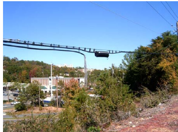
This cable has been hanging since Ivan came through several years ago!
