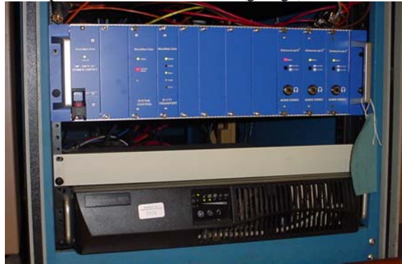
KKPZ's APT Oslo System
