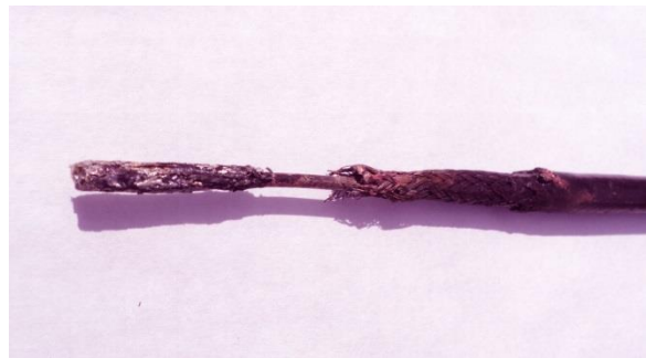
Figure 3 - Cable after removal from entry port.
