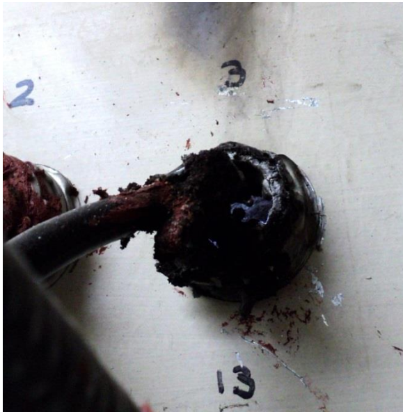
Figure 1 - Cable at building entry port. Note the fire damage.
