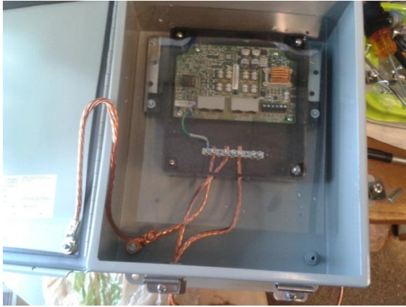
Figure 1 - Now this is how you ground a NEMA box.
