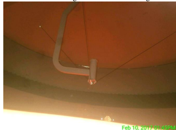
Figure 2 - The crew even looked inside the 8' 'kettle drum' dishes. Everything looked OK.
