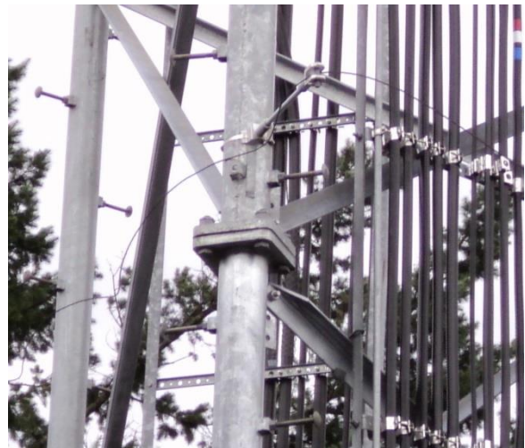
Skirt damage on a nearby detuned tower.
