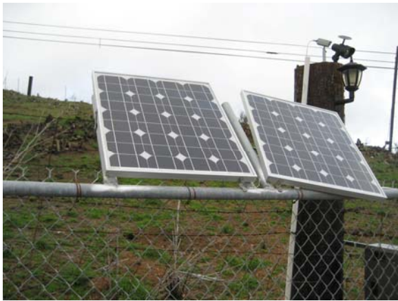
A weld failed on the gate opener solar panel bracket in high winds
