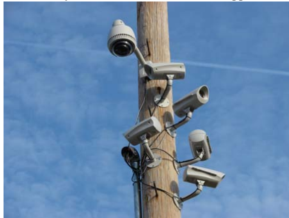
Eyes everywhere... the video surveillance system at the WXJC site includes a dedicated camera on each tower base and a steerable pan/tilt/zoom camera for general surveillance.
