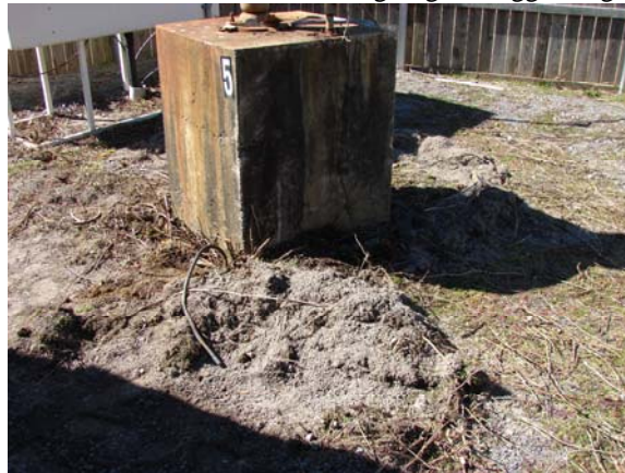
Newly copper-free zone at the base of WXJC tower 5. The thieves even raked up the copper screen under the dirt.
