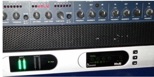
Figure 3 - The new Telos Hx6 in WYDE FM's control room.
