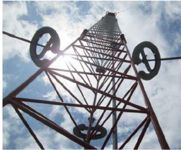
Corona rings installed on top and second from top guy levels on tower 3.
