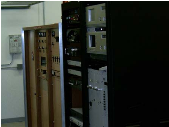
Aux transmitter, digital transmitter and rack equipment
