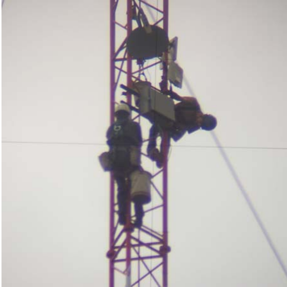
A crew from GRB Construction installs the new Canopy system at KLZ
