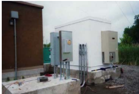
WPWX UPS building
