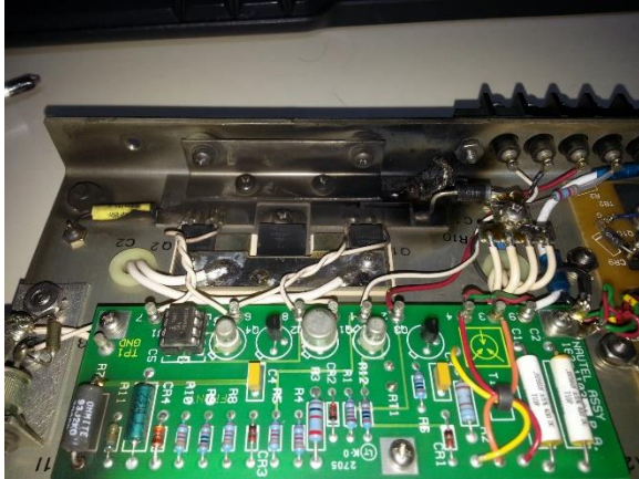
An ND-1 PA module from WEXL that was damaged by high line voltage. Note the blasted modulators and heat damage to R7.
