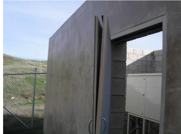
Tower #4 door - before the fix.
