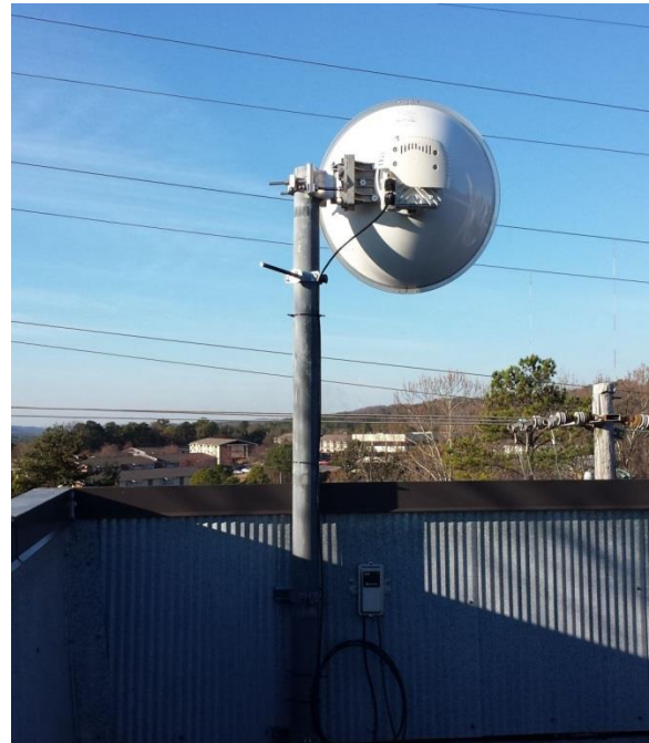
Studio Dragonwave antenna in its permanent location.
