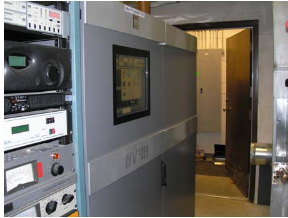
WMUZ's new Nautel NV-40 Transmitter
