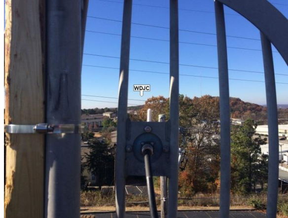
Figure 2 - Now THIS is engineering: the 950MHz backup STL dish temporarily mounted on 2x4s.
