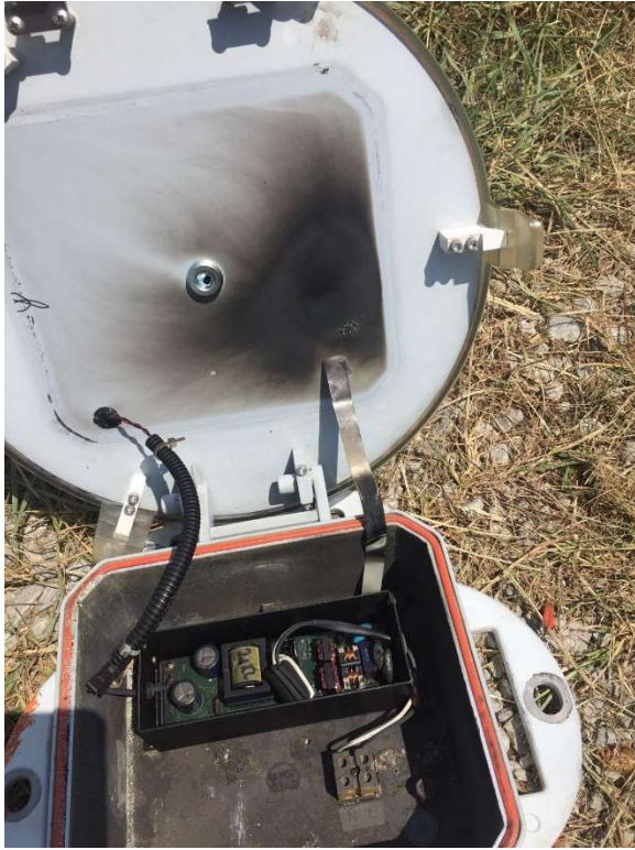
Figure 1 - The smoke escaped from this LED beacon assembly.
