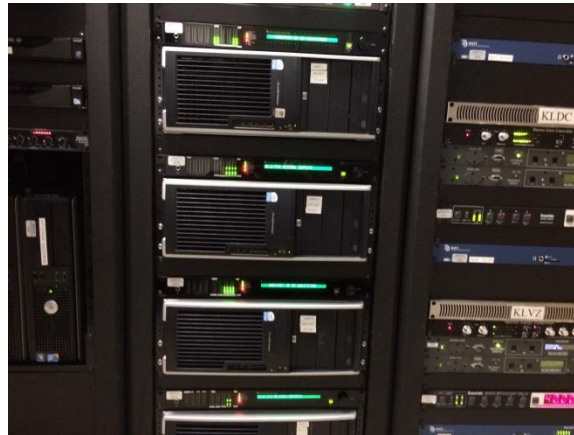
Figure 3 - CBC-Denver's audio server stack with Wheatstone IP blades
