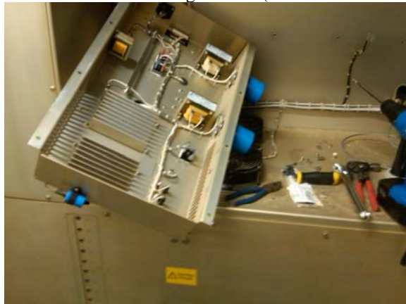
Replacing the fuse holder (on the lower left of the detached panel)
