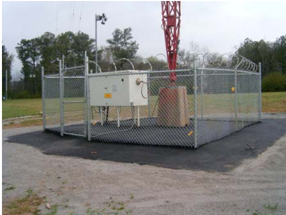
WXJC Tower 3 - note that the fence fabric is sealed in the asphalt
