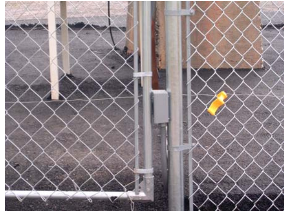
Gate security system switch and lower electric fence wire
